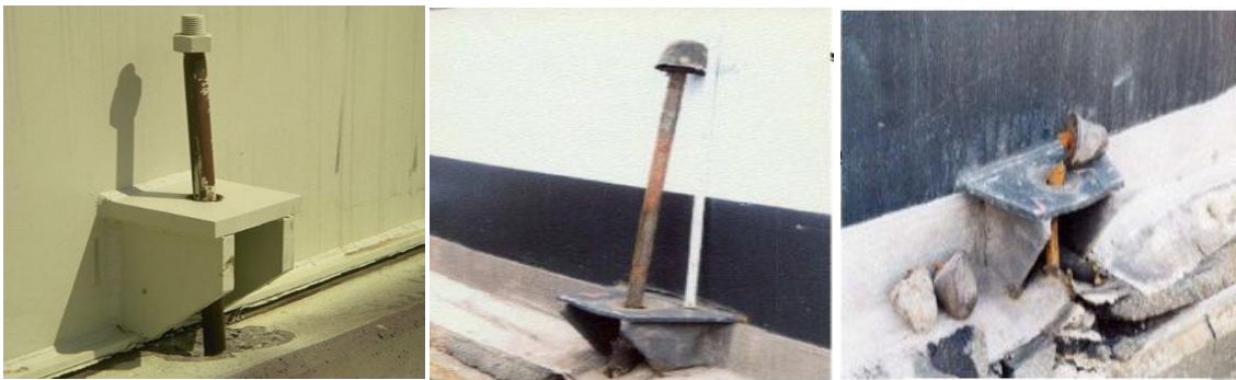
Figure 2. 4 Damage to the anchor bolts and the foundation system (Mohsen and Ali, 2015)
