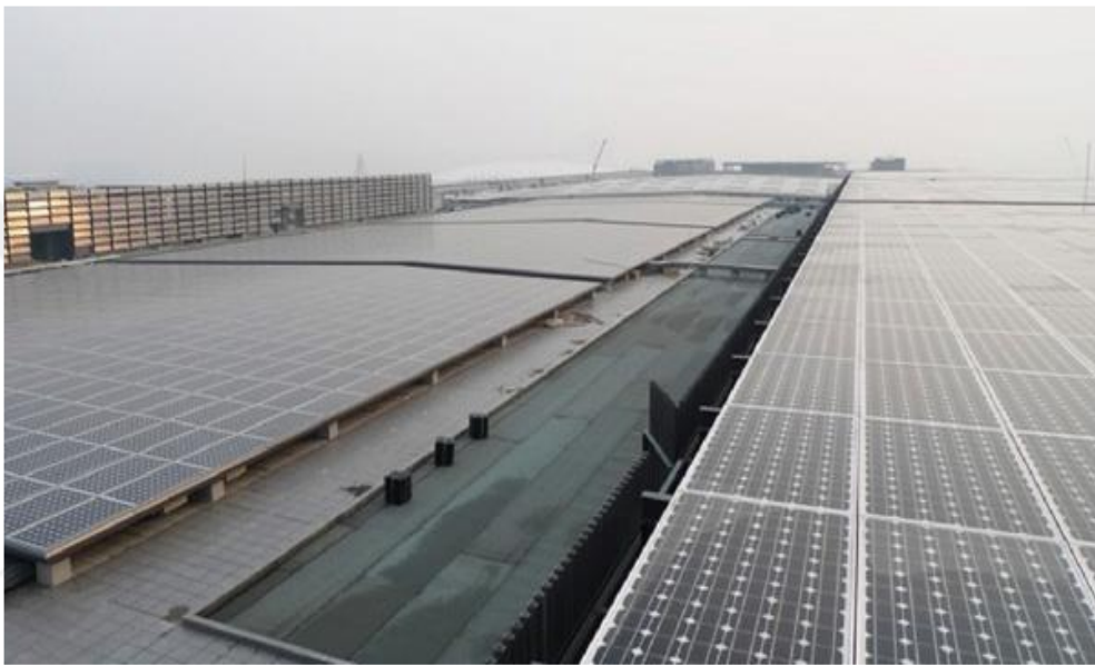
Figure 2.5. BAPV arrays are attached to the roof ( Peng et al., 2011).
