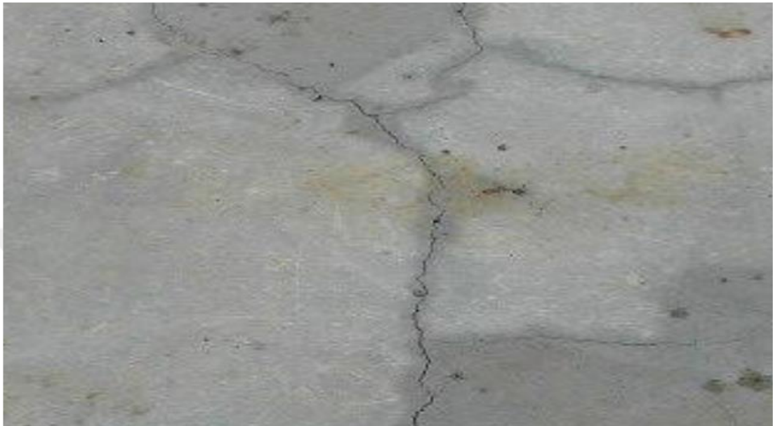
Figure 2.2. Plastic Shrinkage Cracks
