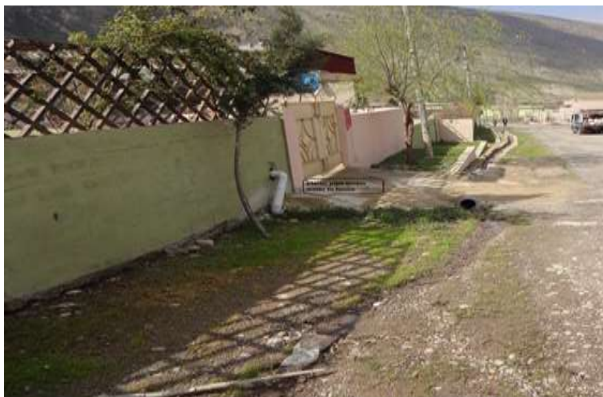
Figure 4.8 Plastic connection pipes from network to village houses
