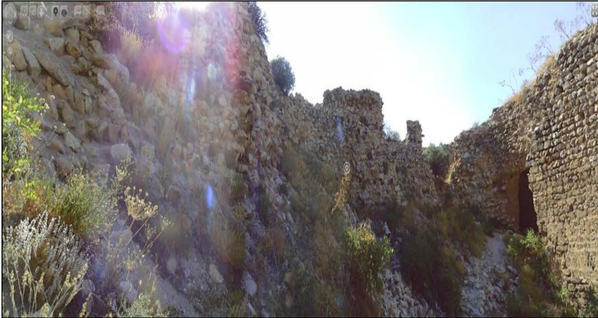
Photo 5. View of South Wall Interior Wall Problems
