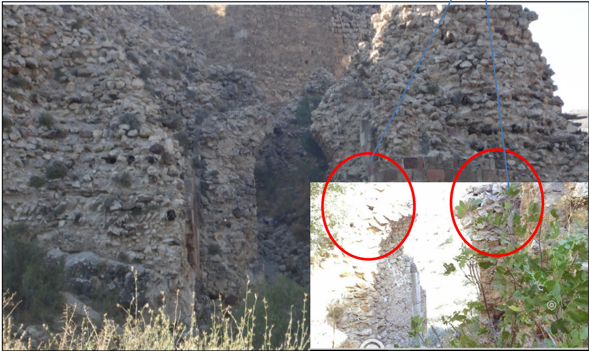
Figure 12. North Wall, Main Entrance Door Exterior Wall Completely Lost and Belt Destroyed
