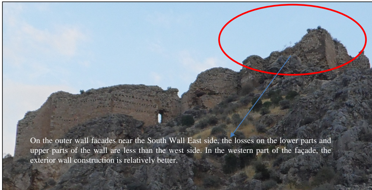
Figure 6. General representation of structural problems of southern wall
