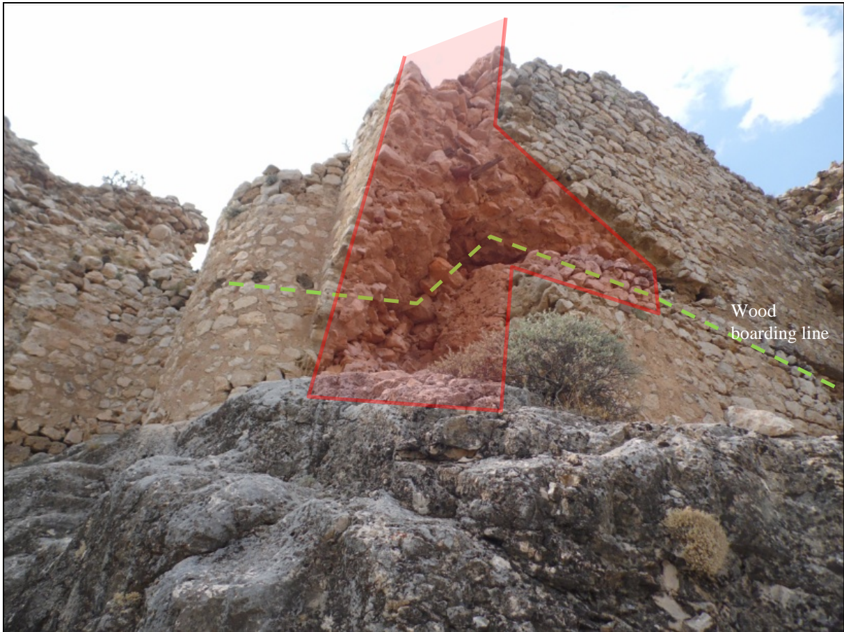
Figure 7. Bottom Wall Discharge at Southern Wall Wall GD-8
