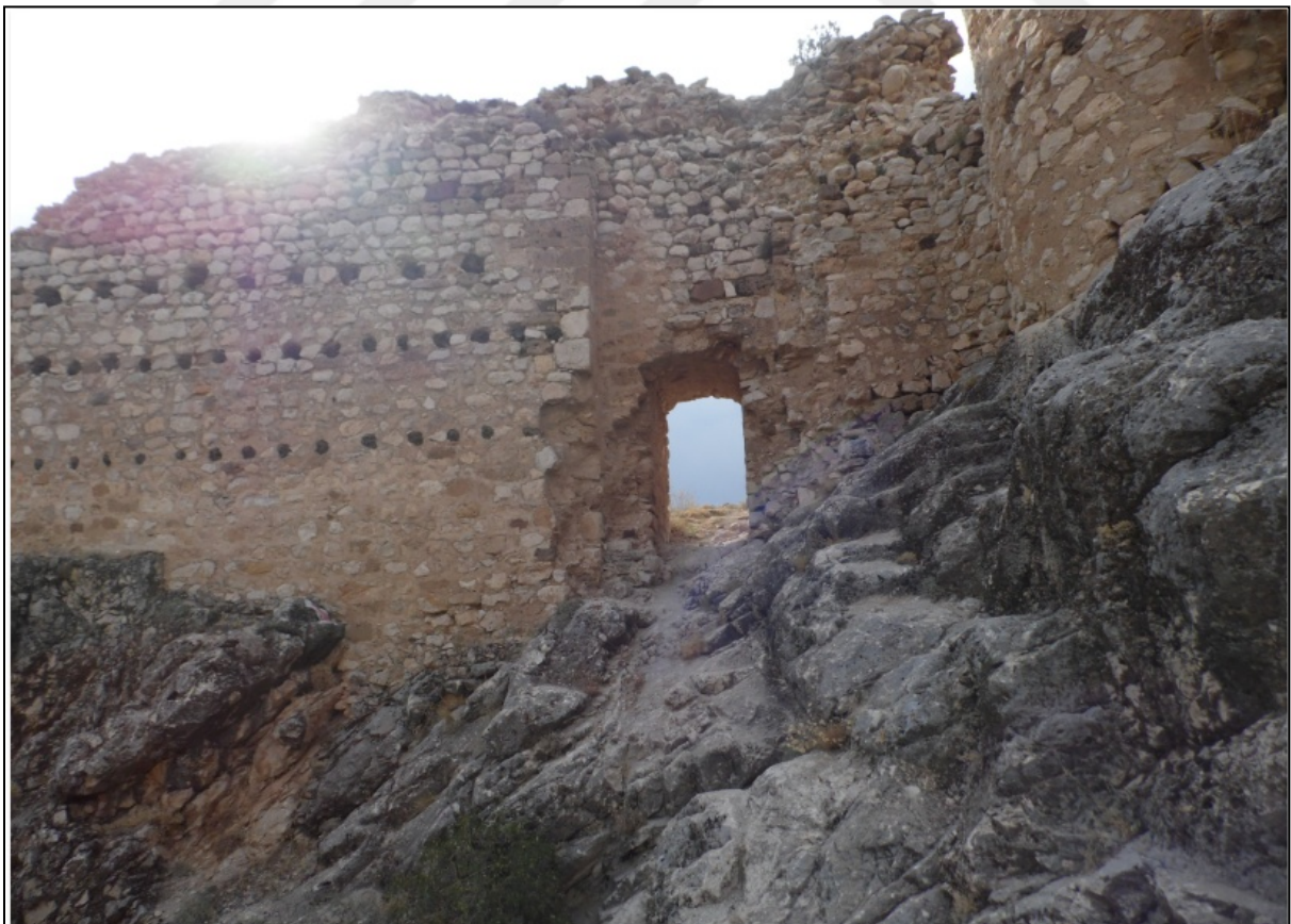
Photo 4. Knitting Stone Loss Around the Entrance Wall of the South Wall
