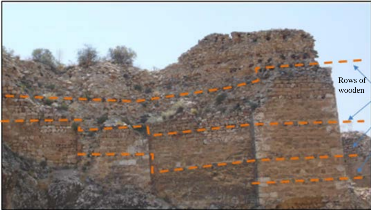
Figure 10. Close view of the walls between the North Wall and the KD11-KD17
