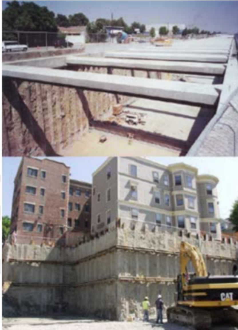
Figure 2.19: Top: Trench excavation railroad for an Alameda corridor project. bottom: Structural cut-off wall during construction of new facility at Harvard University, Cambridge (Porbaha et al., 2005)
