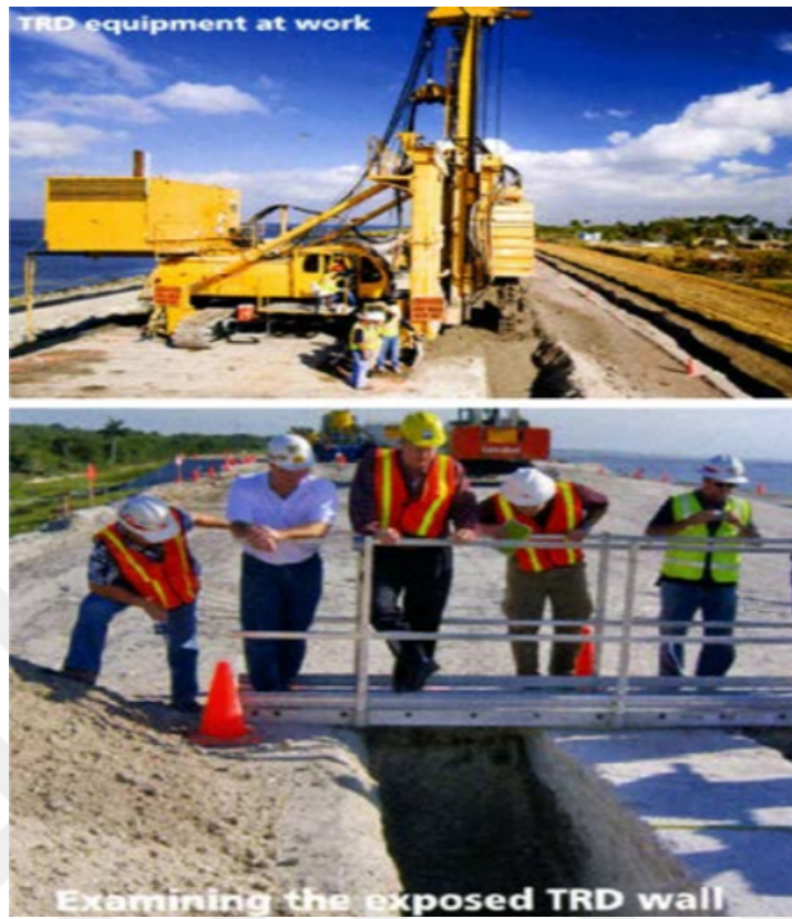
Figure 2.17: Top: TRD equipment at work, bottom: Inspection of the exposed TRD wall at Herbert Hoover Dike surrounding Lake Okeechobee in south-eastern Florida (Inc., 2012)
