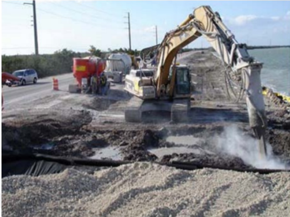
Figure 2.27: Dry mass soil mixing to strengthen soft soils beneath a planned roadway expansion at U.S. Highway 1, Key Largo, Florida (Inc., 2012)
