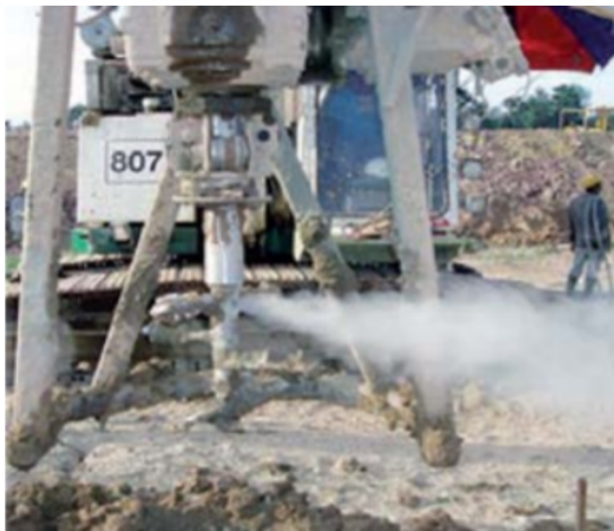
Figure 2.12: Injection of dry binder into the soil from the mixing tool (Keller, 2011)
