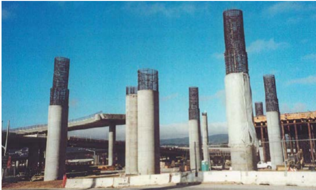
Figure 2.14: Railroad bridge supported by deep mixing column at San Francisco International Airport (Porbaha et al., 2005)
