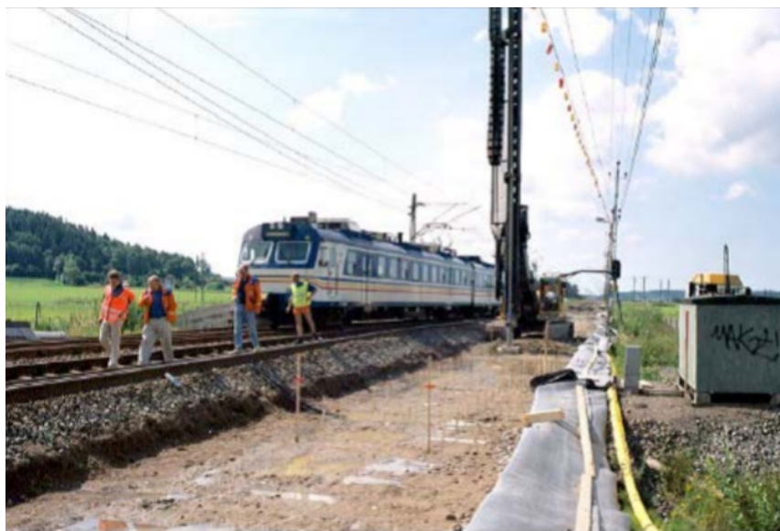
Figure 2.22: Vibration mitigation using dry deep mixing method; column installation in progress while commuter train passing (Holm et al., 2002)
