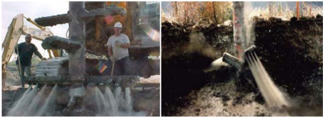
Figure 2.6: Parts of wet mixing tool showing injection of slurry into the soil (Porbaha et al., 2005)
