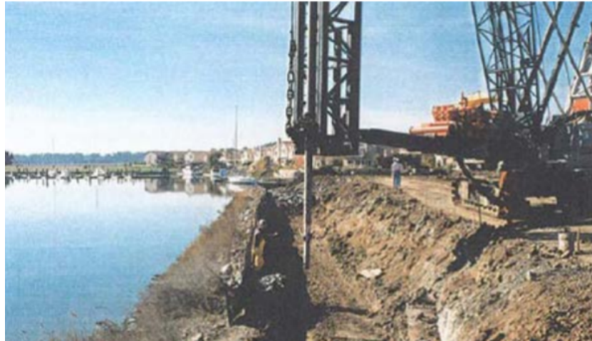
Figure 2.23: Liquefaction mitigation along river bank at Napa Yacht club, California (Porbaha et al., 2005)
