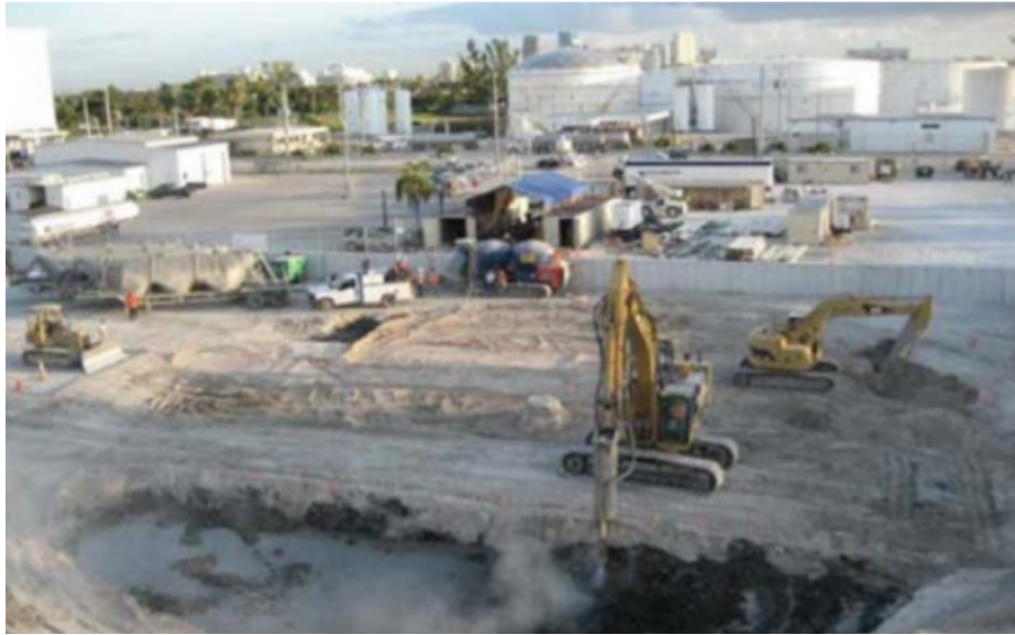
Figure 2.28: Mass stabilisation with dry soil mixing of soft wet organics to control settlement for storage tanks at Port Everglades, Florida (Inc., 2012)
