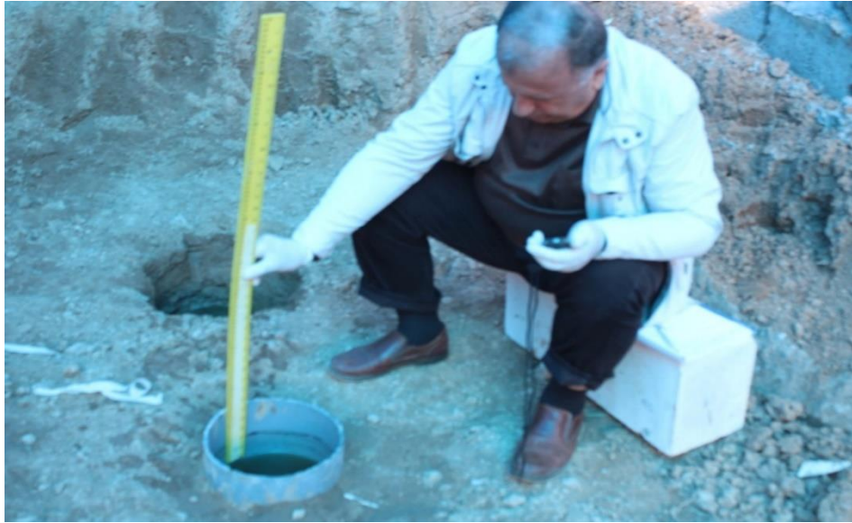
Figure 5.14 Penetration pits for oily wastewater.
