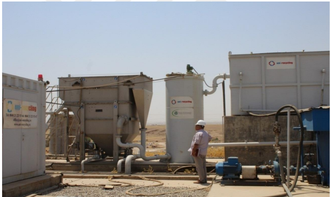
Figure 4.4 Kawergosk wastewater treatment plant.
