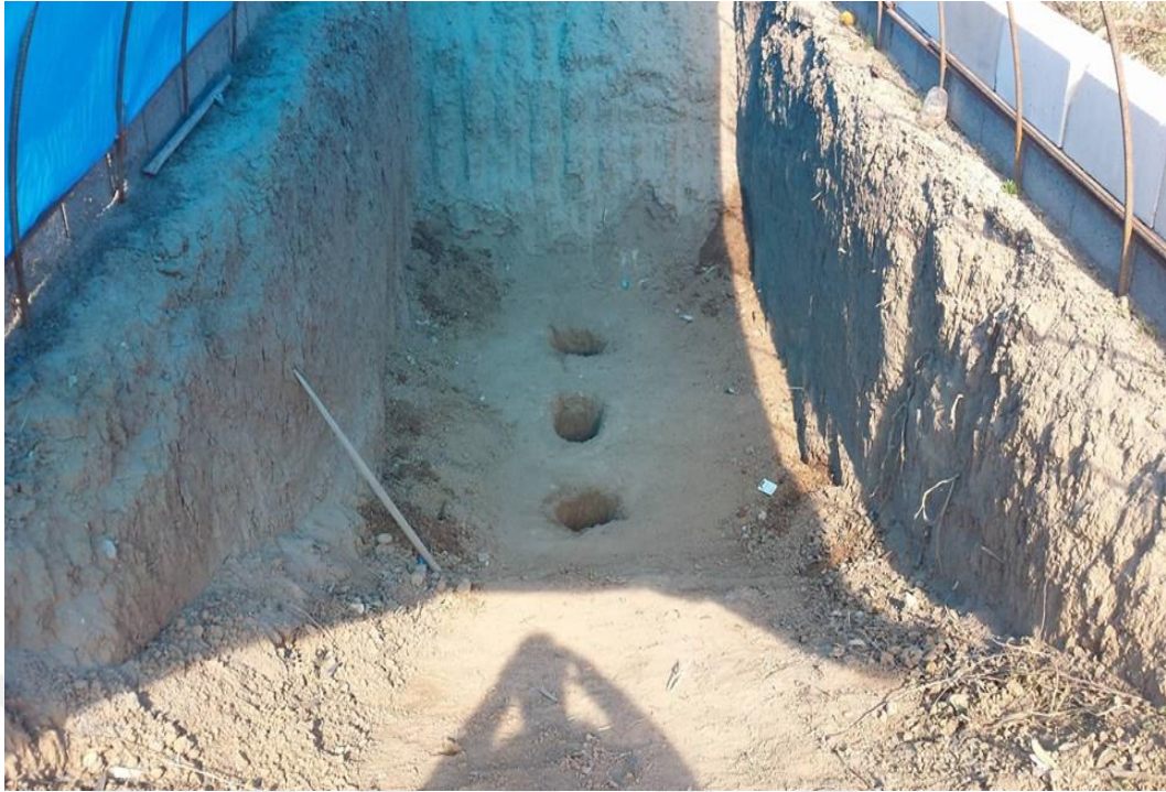
Figure (4) Field pit.
