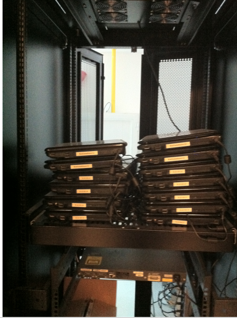
Figure 8: Laptop Cluster in Data Center.
