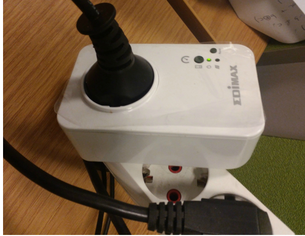
Figure 16: Power meter is connected between the main computer and plug
