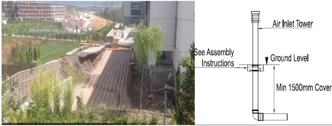
Figure 3. 7 Construction stages of the underground heat exchanger and the sensors being added inside pipes.
