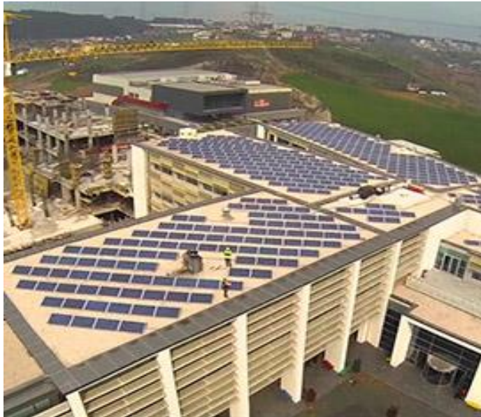
Figure 3.10 PV panels on the roof of the building
