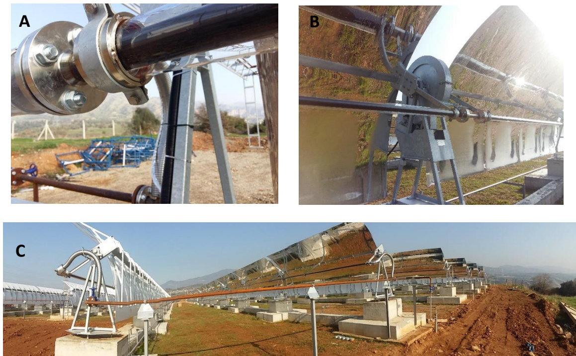
Figure 6.2 A-the connection absorbers, B-the tracking system, and C-the solar field.
