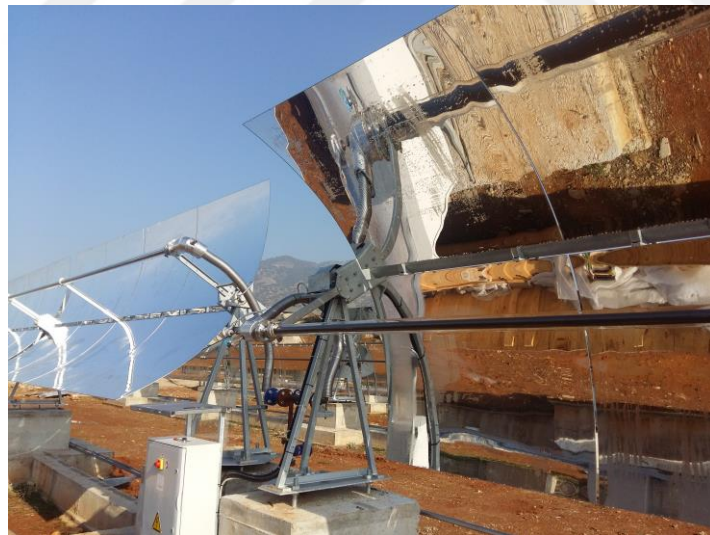
Figure 1.2 Receiver and reflector for PTC system (This project is at the campus of Adnan Menderes University, Aydin, Turkey, which was built with the help of the European Union FP7 BRICKER project and manufactured by Soltigua of Italy).
