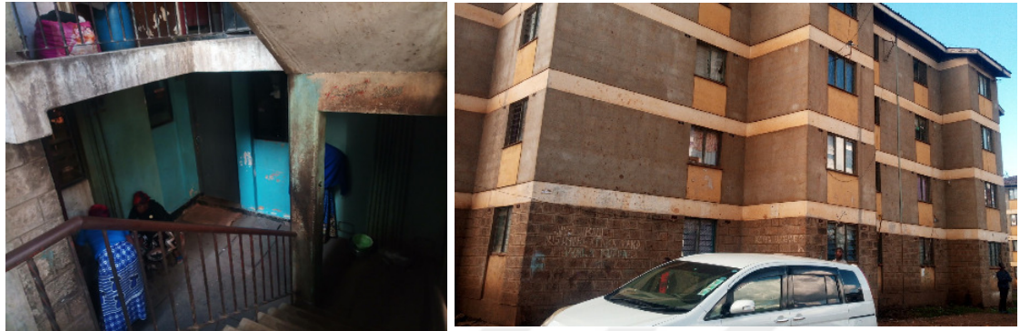
Figure 4.33 and 4.34: Evidence of vandalism like graffiti and lack of maintenance on structure walls in Pumwani-Majengo
