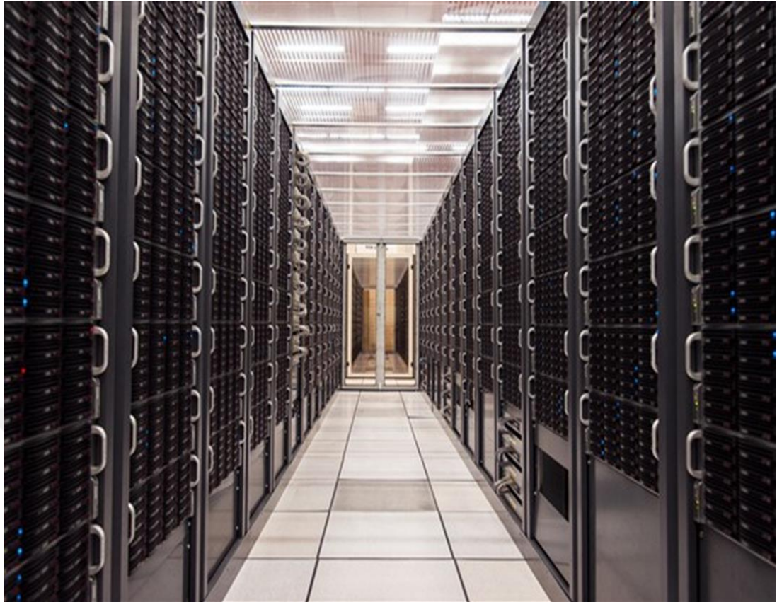
Figure 1.11. Computing Center - CERN.
